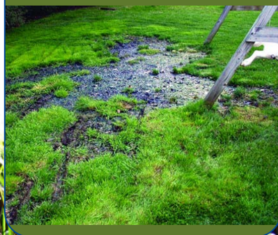
Effluent from a failed drainfield has surfaced in this backyard.
