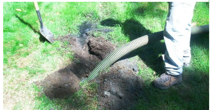
Ponded Effluent Removal from Leachfield
