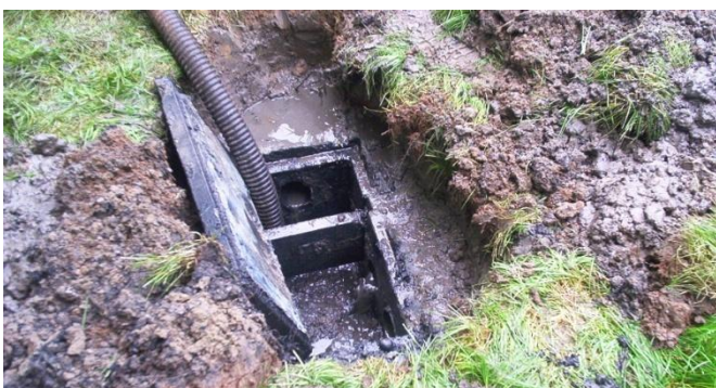
Ponded Effluent Removal from Distribution Box
